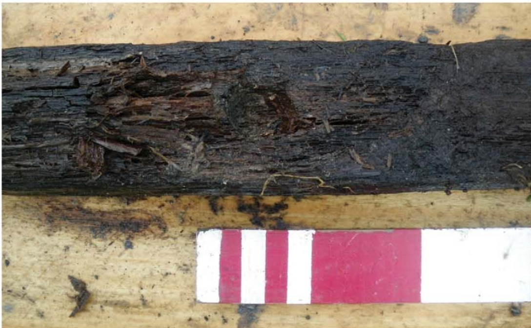
Plate 28: Detail of dowel hole in Timber 64. Scale 0.15 m
